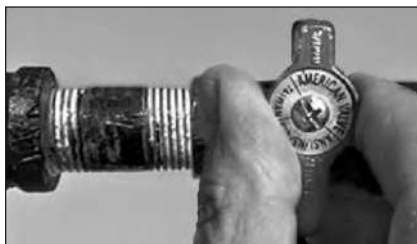
Figure 37 - Manual Gas Valve in OFF position.
