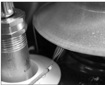
Figure 26 - Test the air supply and vent to make sure the water heater has adequate air and is venting properly.
