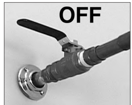
Figure 11 - Cold water supply in OFF position.
