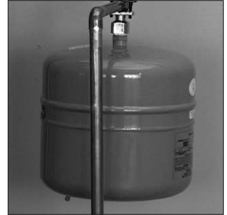
Figure 19 - The Thermal Expansion Tank should be pressurized with air, to match the home's incoming water pressure.
