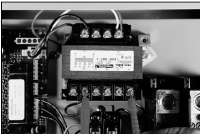
Primary Winding Voltage Test
