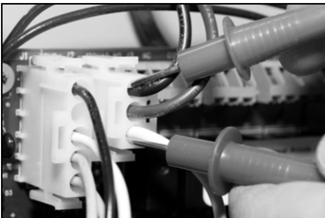
Checking for 120 VAC
