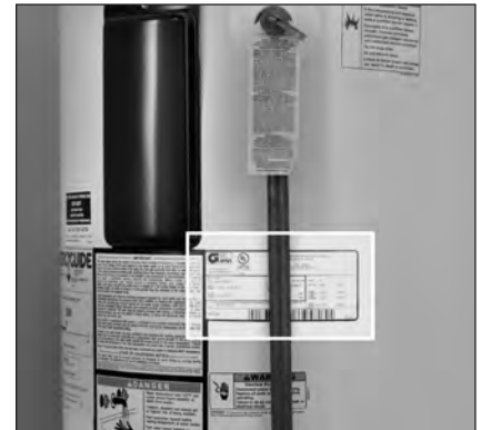
Figure 18 - The water heater’s electrical requirements can be determined from the data plate.
