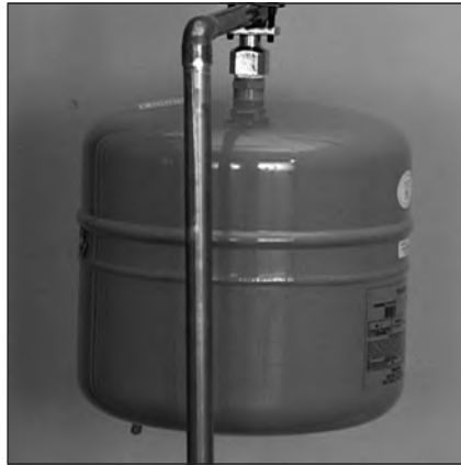
Figure 16 - The Thermal Expansion Tank should be pressurized with air to match the incoming water pressure.
