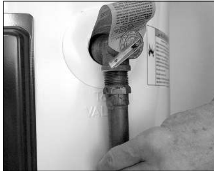
Figure 12 - The T&P Relief Valve discharge pipe must be installed properly and piped to an adequate drain.
